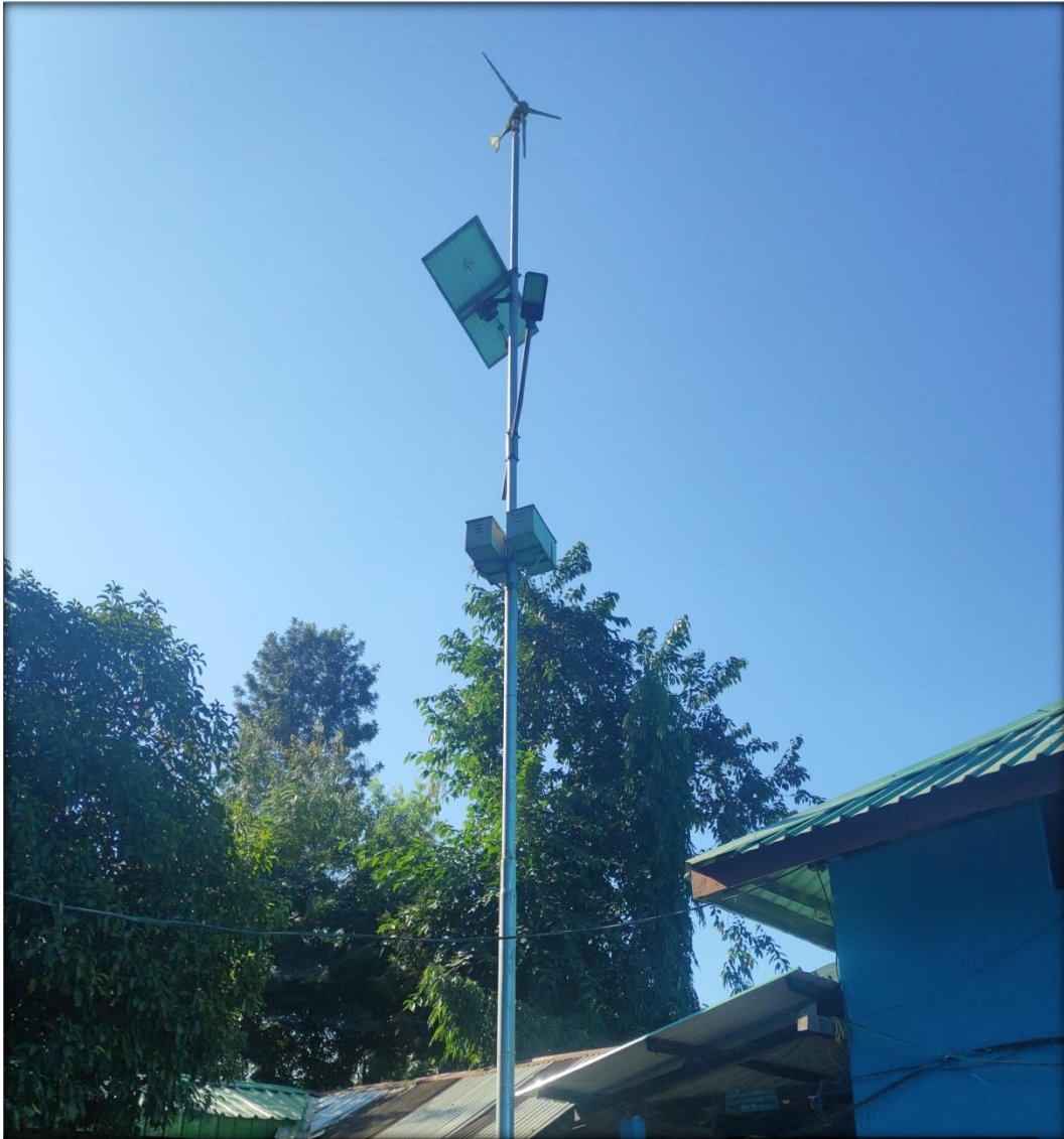
Fig 14: A LED Wind Solar Hybrid Street Light
